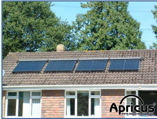
Installation chauffage solaire (88 tubes)
